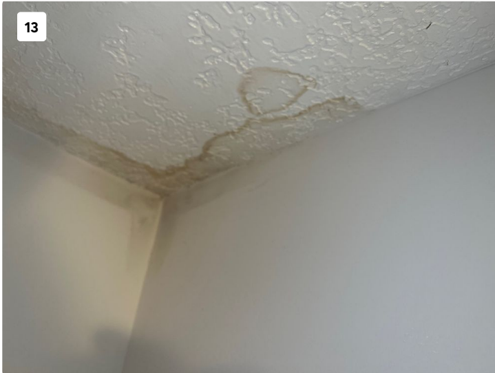
Water damage on the ceiling indicates water intrusion from the chimney.
