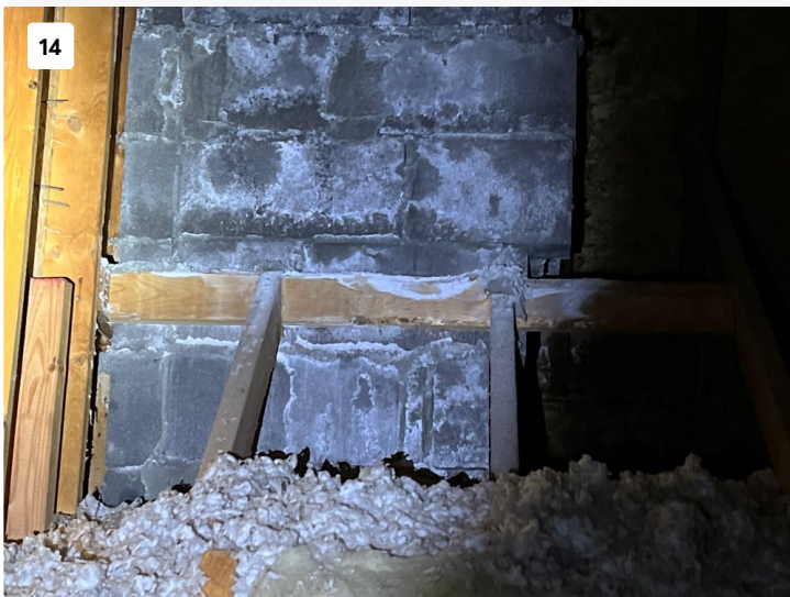
This picture is taken in the attic. The white stain is efflorescence. This is evidence of water intrusion. The stain is the salts and minerals that the water is picked up from the masonry and deposited here as it dried.
