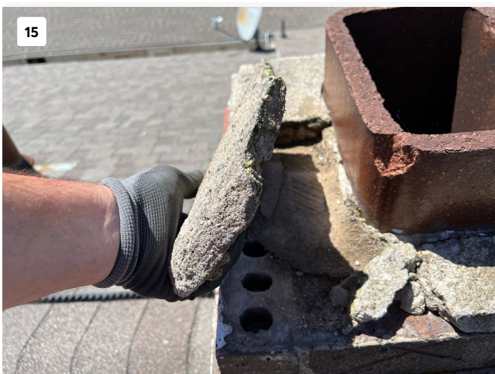
The mortar wash on top does not adequately protect the chimney from water intrusion. It should overhang the face of the chimney to provide a drip edge keeping a majority of rain water off the face of the chimney. This is such a bad condition that parts of it can be removed by hand.
